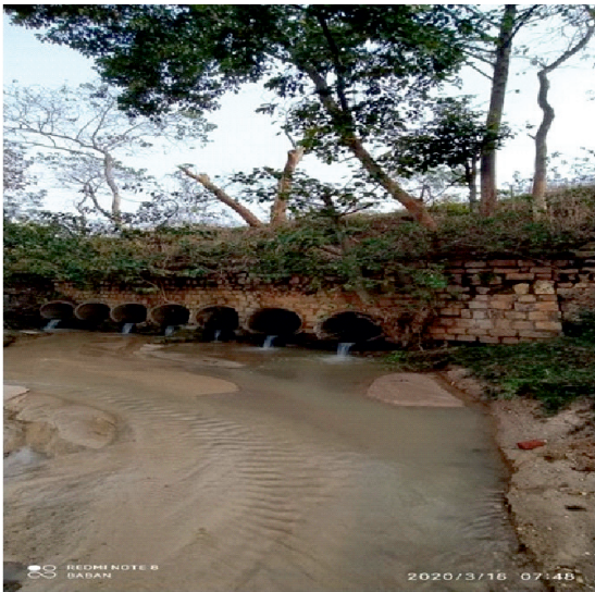
Figure 7: Soil Erosion at Bantoli
